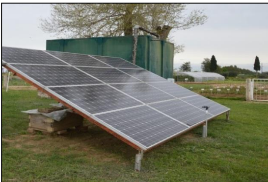
Solar Pumping System (2600 Watts) linked with HEIS
